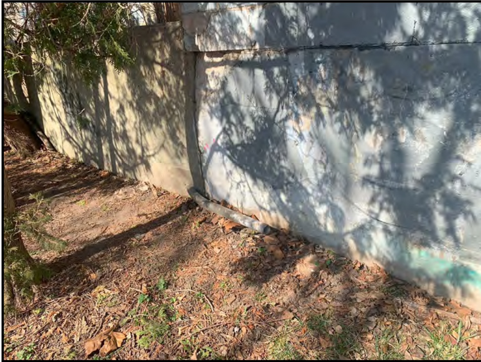
Photo 17: View of a metal pipe located beneath the former 10,000-gallon UST observed along the southern border of the subject property building.
