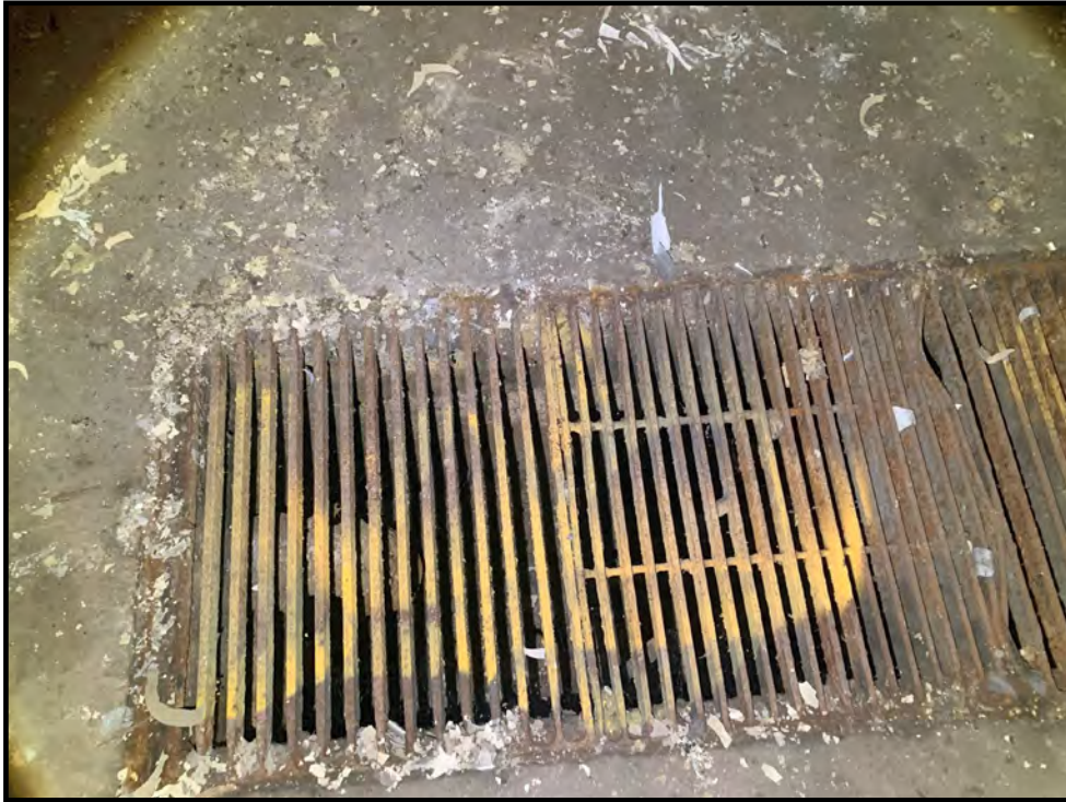
Photo 7: View of the trench drain within the southern portion of the subject property building.
