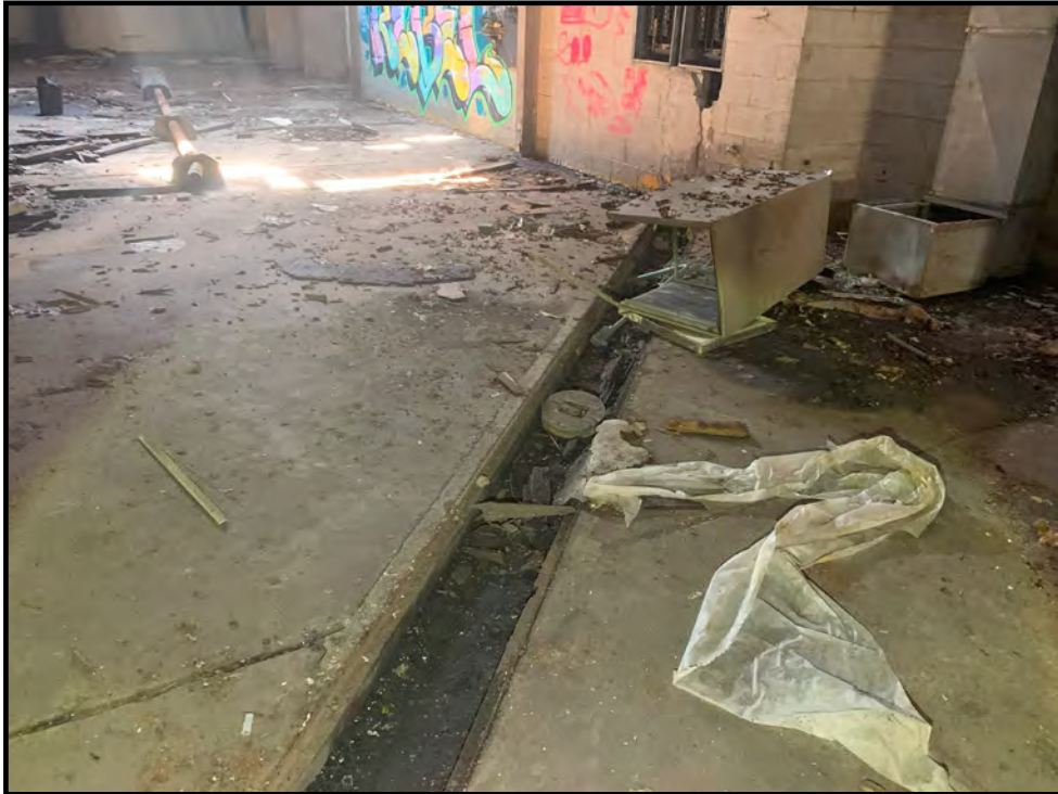
Photo 13: View of the trench drain observed in the northwestern portion of the subject property building.
