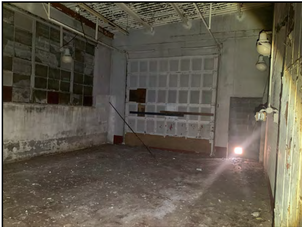
Photo 6: View of the garage door located at east side of the subject property building.
