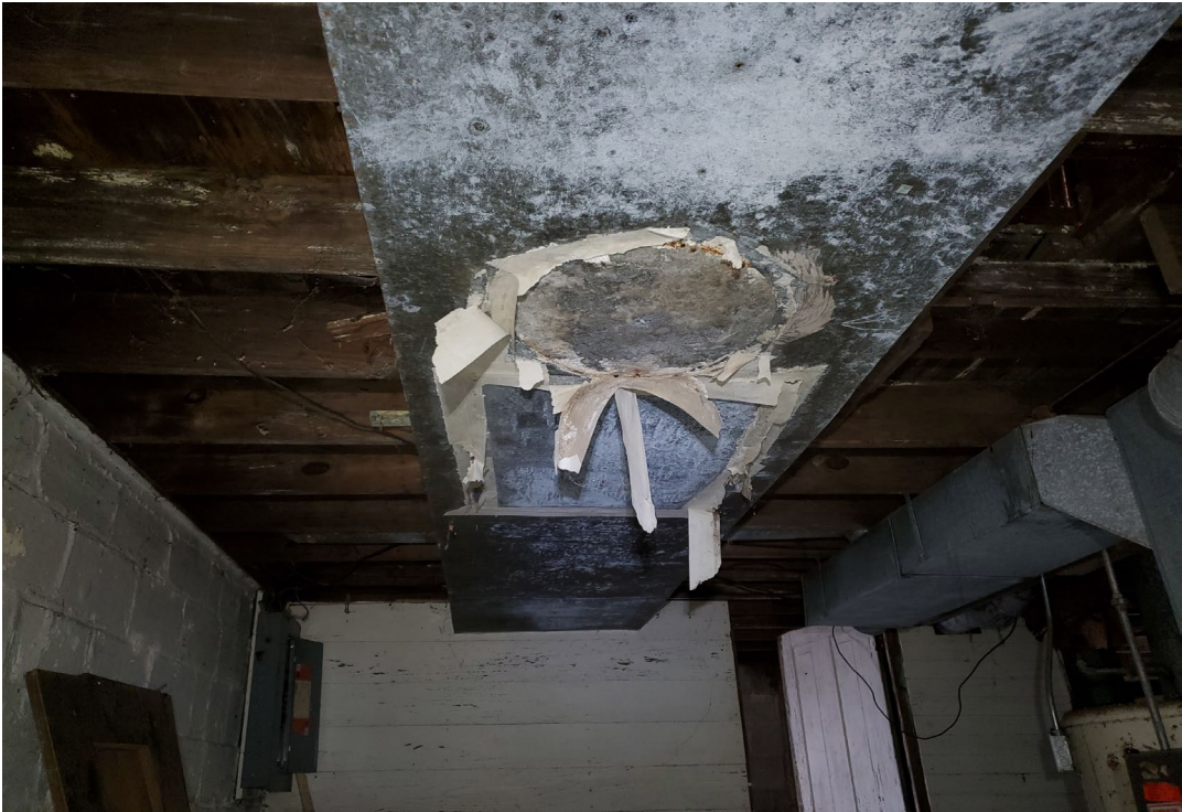
PHOTO: 4 SUBJECT: Basement HVAC Tape on Duct and Framing
