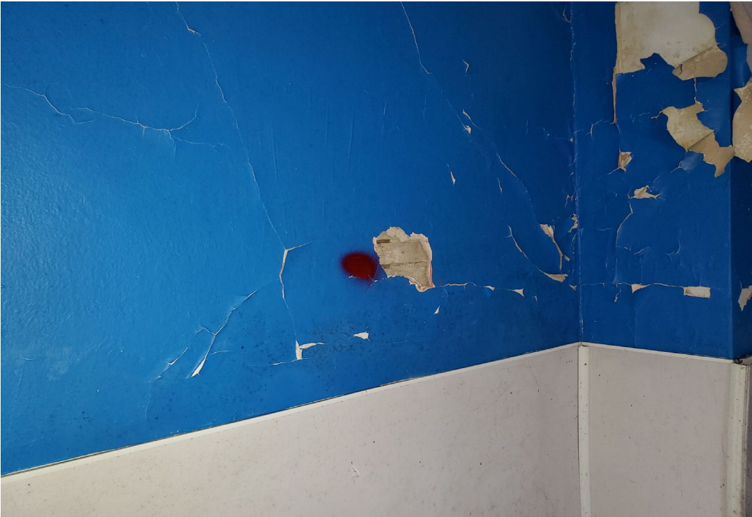
PHOTO: 6 SUBJECT: Kitchen Wall Plaster
