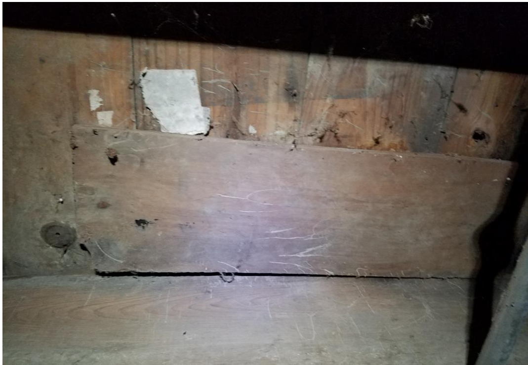
PHOTO: 6 SUBJECT: HVAC Paper on Basement Framing
