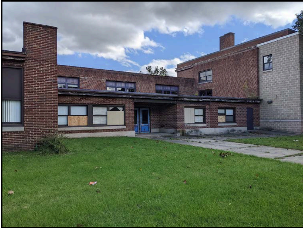
Photo 3: View to the southeast from the northwest corner of the subject property.
